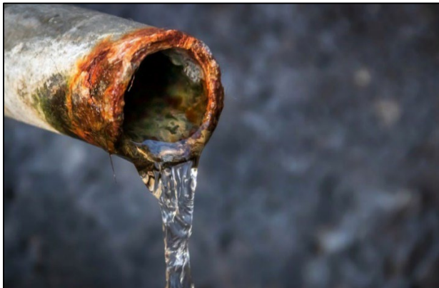
Corroded Lead Pipe. Source: Creative Commons
