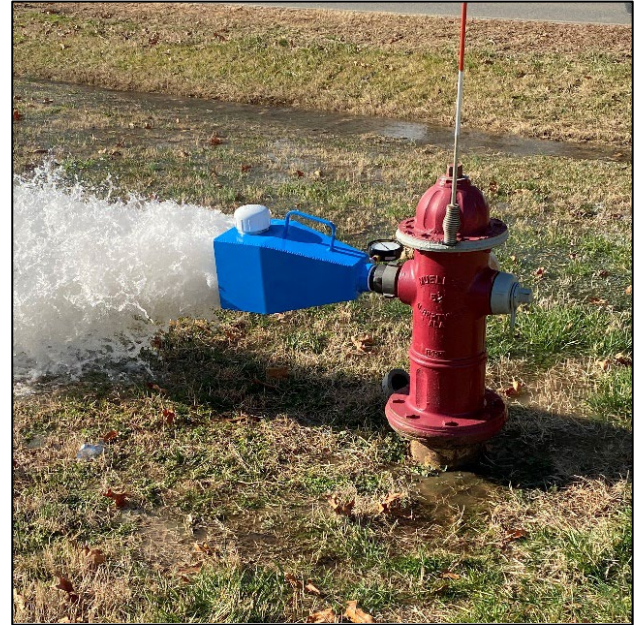
Fire Hydrant Flushing at Naval Support Facility Dahlgren. Source: NSFDL Stock Photo
